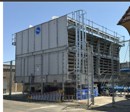
New Cooling Tower
