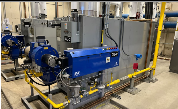
New Gas Boilers
