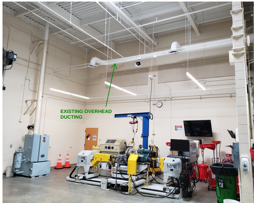
OVERHEAD RELIEF DUCTING & VENT AREA
