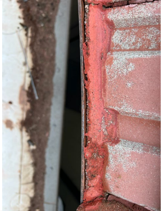
Red Seam Sealant at Tile Roof
