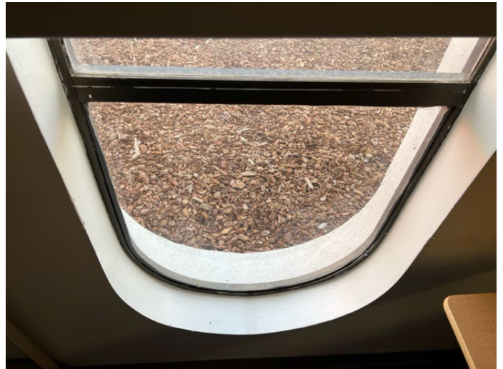
Brown Window Frame Sealant-Asbestos & PCB
