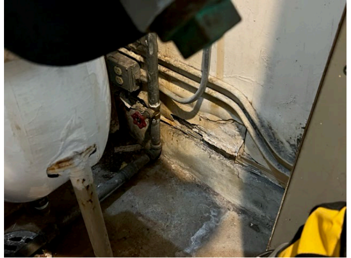
Delaminating Sheetrock with Mold in Mechanical Room
