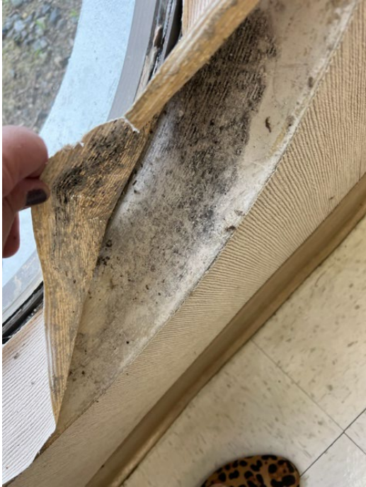
Mold Found Behind Wallpaper in Classroom
