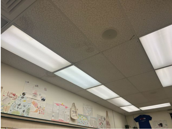
2'x4' False Ceiling Panels-Old -Asbestos
