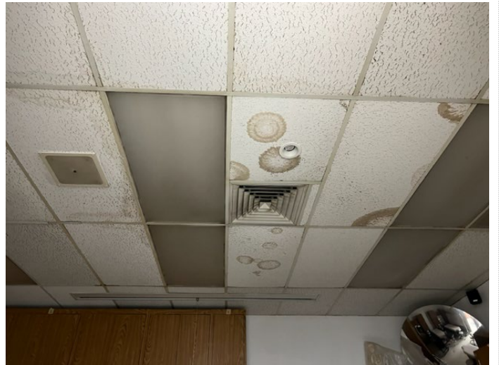
Water Leaks found in Classroom
